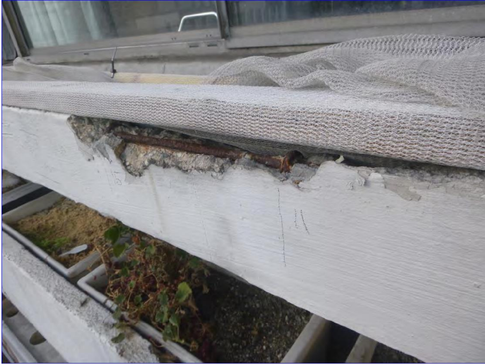
Photograph 5: South Elevation, Cullum Welch House. Close up view of planter and pot holder showing spalled concrete and exposed rebar after removal of loose material.
