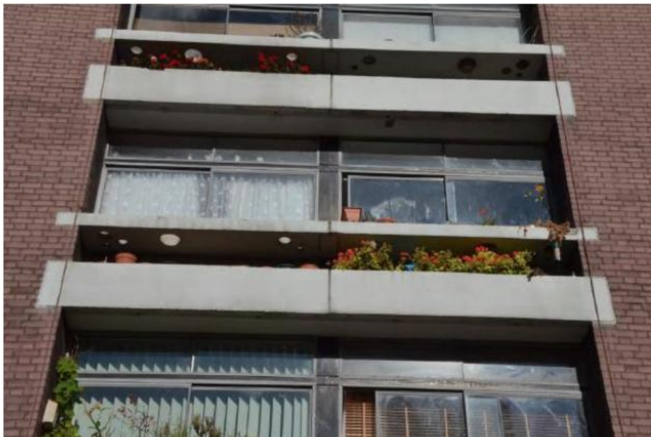
Photograph 4: South Elevation, Cullum Welch House. View of typical windows planters and pot holders which span two dwellings (partition wall at the centre of the view). Photograph was taken before the installation of safety netting.
